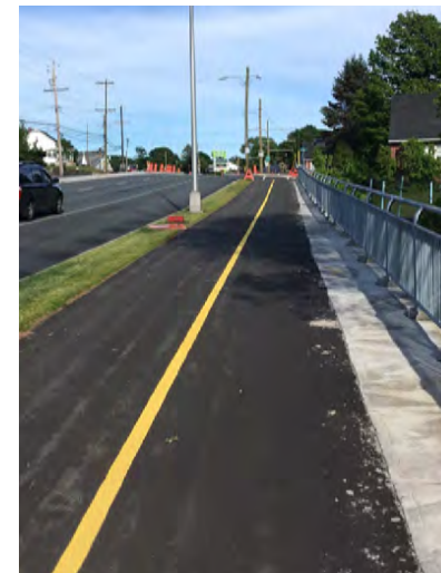
Mixed-use Pathway adjacent to an arterial roadway, including a fenced portion for an incline.
