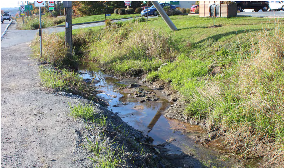
Ditch between Trunk 7 and Tim Hortons parking lot
